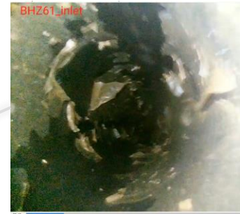
Inside cooling hose. Analysis: ( https://edms.cern.ch/document/3064730 )
