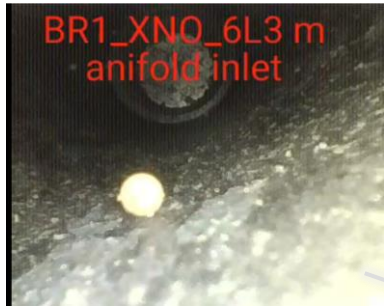
Demin Resin in the inlet manifold
