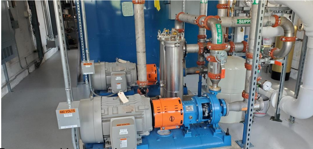
Pumps and heat exchanger
