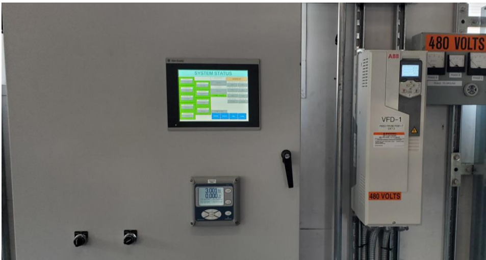
Controls and VFD
