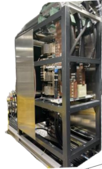
Circuit disconnecter boxes
