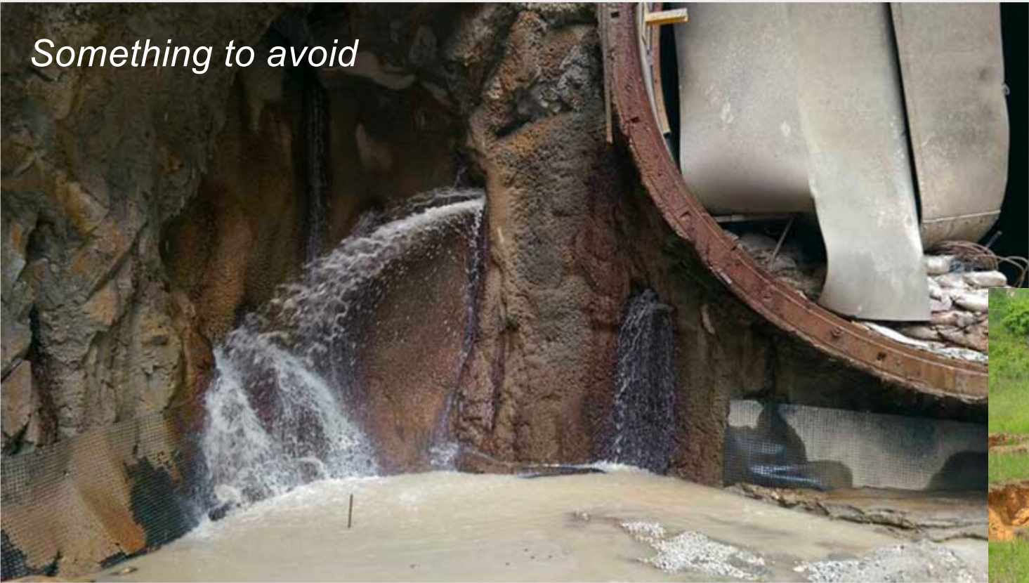
Water inrush through the end wall of the Pasar Rakyat station box from a network of karst features
