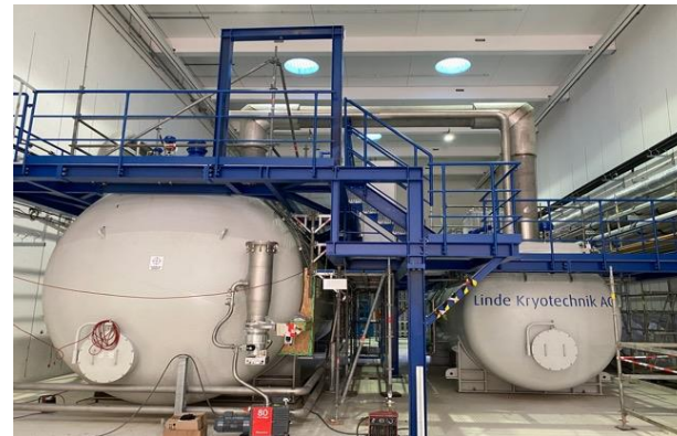
Helium tanks of cryo facility installed
