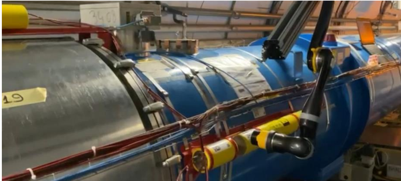
Robotic arm performing a BLM Calibration
