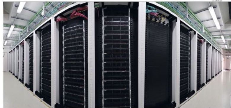
New nodes The event processing node racks in the ALICE computing farm, part of a completely new computing model for Run 3 and beyond.
