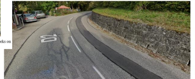
The wall on the inner side of the curve could represent a problem for the convoy; the best path shall be analysed in detail and a modification of the wall may be necessary.
