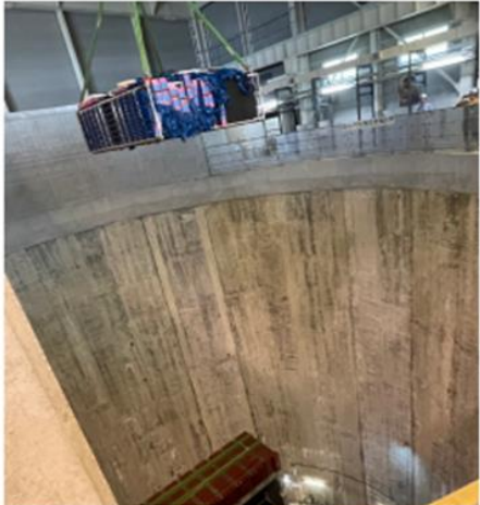
Super-FGD installation (October 2023)
