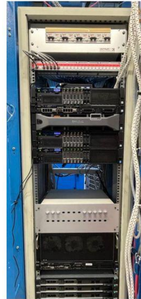
Level-1 Data Scouting rack
