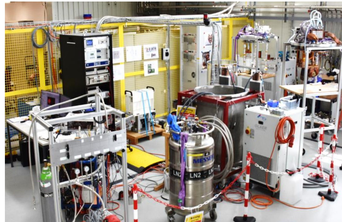
Test station for conduction cooled magnets
