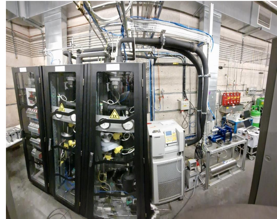
R134a recuperation plant installed at CMS
