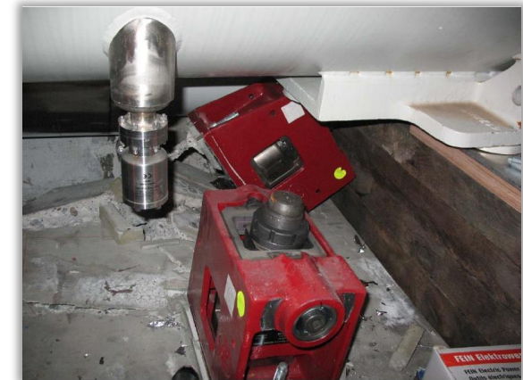
LHC jacks ripped from the ground
