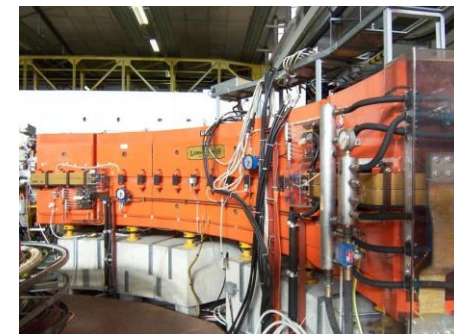
LEIR main dipole, 60 tons
