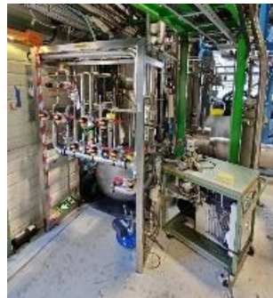
Gas management panel
