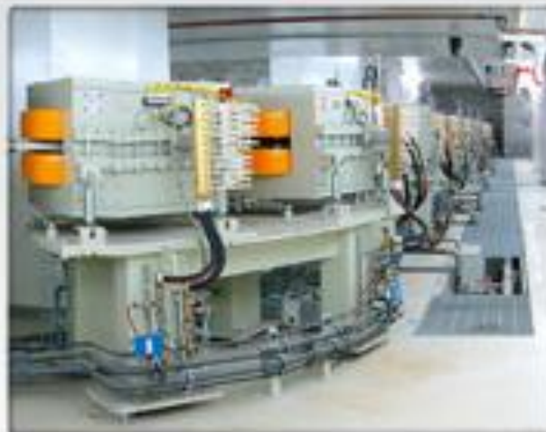
Beam Transport System
