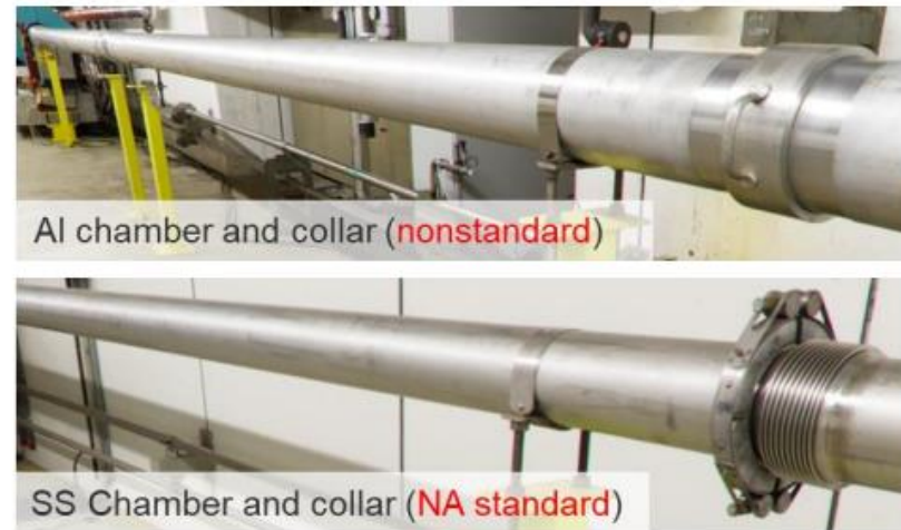
Figure 2: Non-standard vacuum chambers of the M2 beamline compared with the standard stainless-steel chambers used in the other North Area beamlines.
