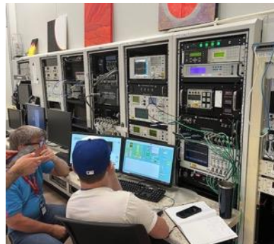
8/26/24: FNAL VTS Control Room
