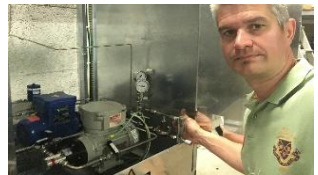
Frederic Gas & Cooling workshop Spare parts (mechanical)
