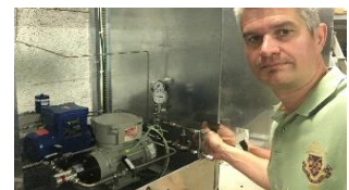
Frederic Gas & Cooling workshop Spare parts (mechanical)
