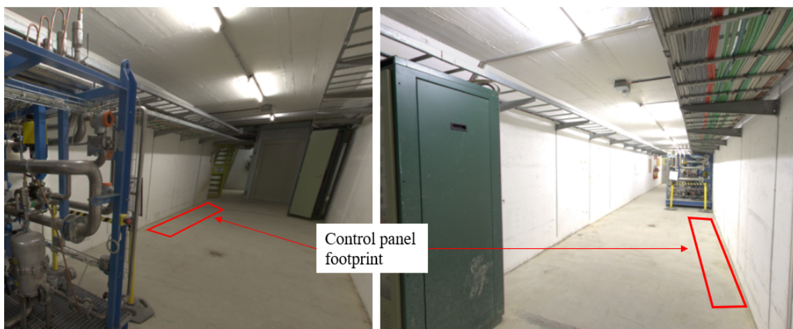
Figure 11 – Pictures of the TA851 tunnel with the designated position of the control panel
