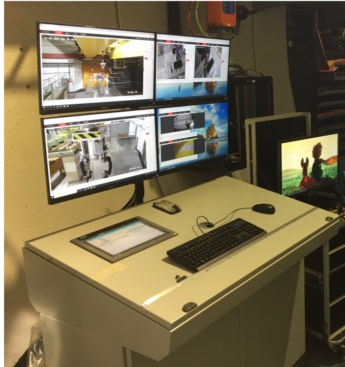
Figure 18 – Example of operator desk
