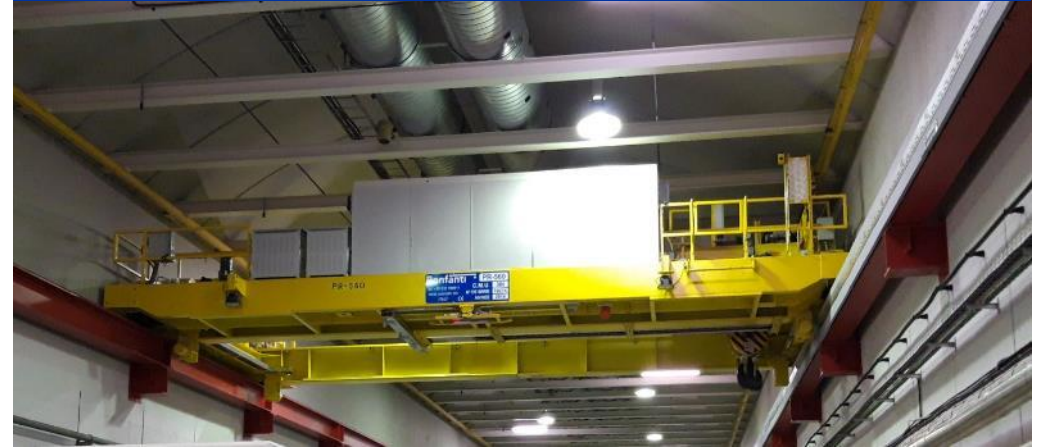
Current overhead crane in TCC8
