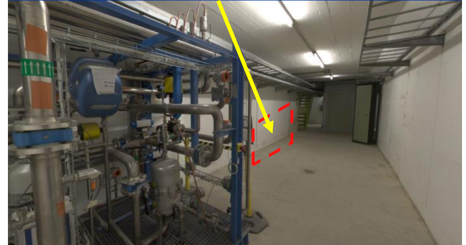
Control panel location in PP851
