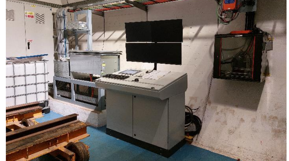
Operator desk in a similar installation
