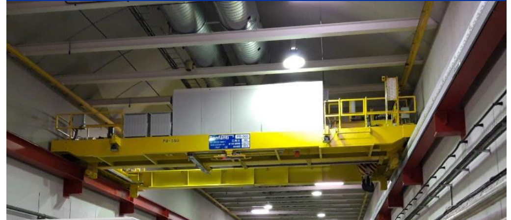
Current overhead crane in TCC8
