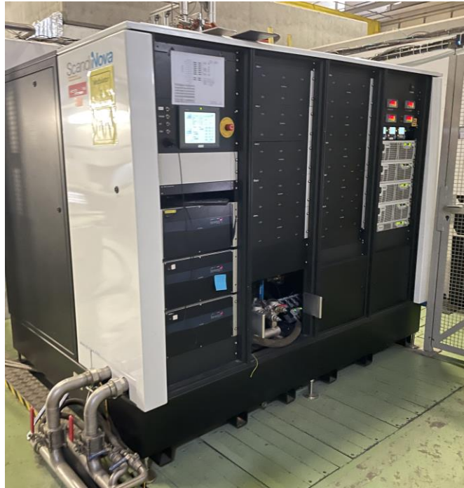
Refurbishment of ScandinoVA modulator to improve operation at higher voltages
