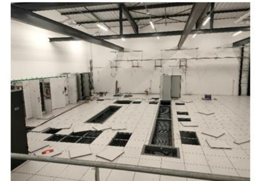
Power supply room
