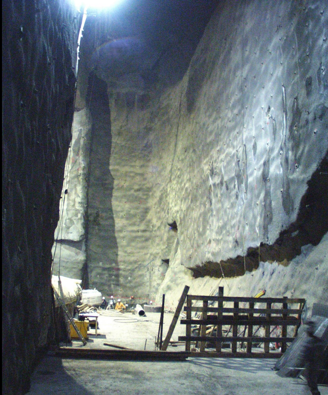
Point 5 - Shuttering for the first layer of pillar concrete - April 20, 2001 - CERN ST-CE
