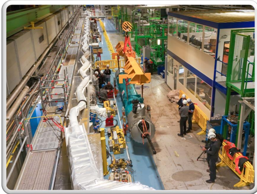
D1 installation and sc link
