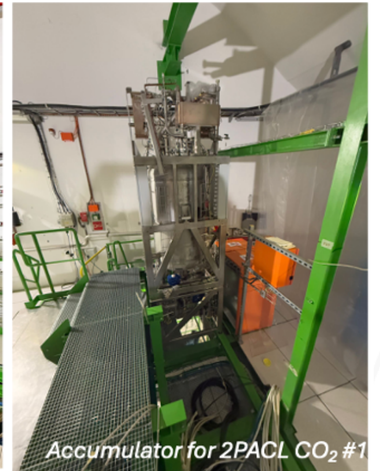
2PACL CO 2 plant #2
