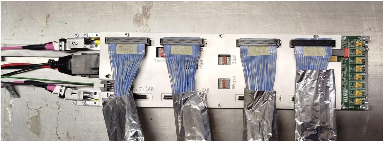
Figure 12 -The OB DT board, connected with power and Front End cables, and optical fibers going to backend electronics.
