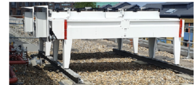
Dry air cooler 2 x 300 KW, PUE 1.3*
