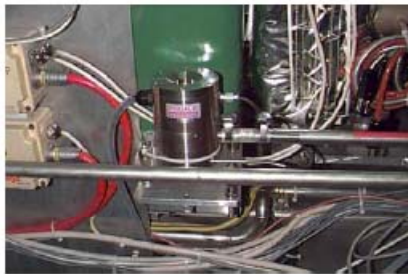
Hydrostatic Levelling System (HLS)
