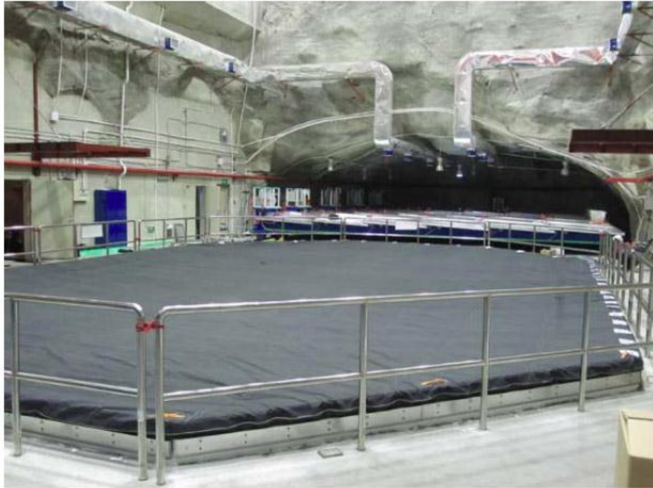
Filled pool cover on
