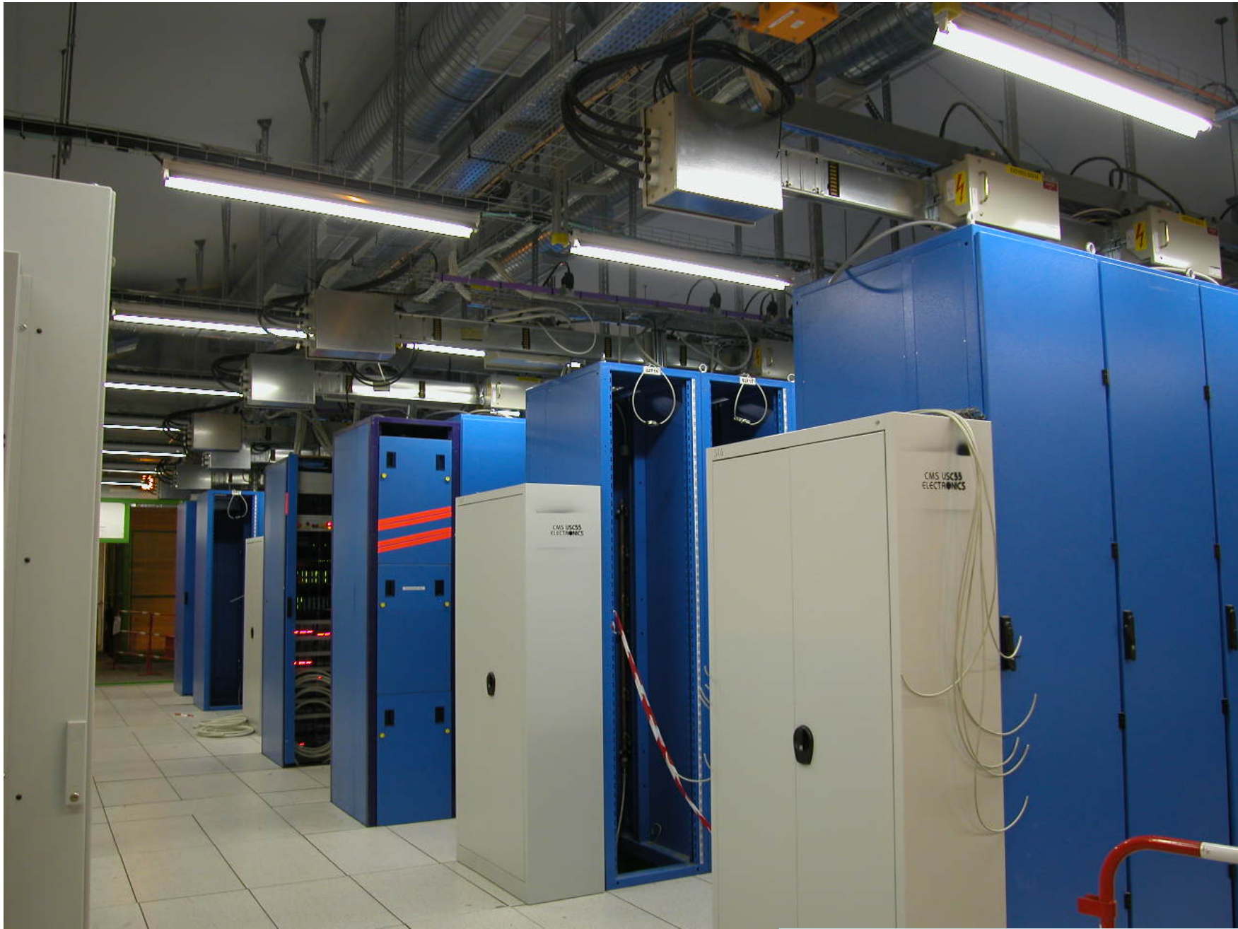
USC55 Rack Room
