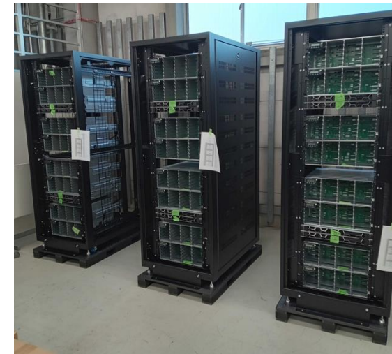
Server rack for storage
