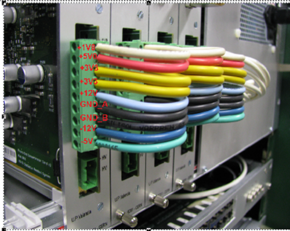
Figure 2 Color-coded power bus cable for 4 Combos, daisy chain connected to 9way Phoenix TMSTB power connectors. All cables have 2.5mm 2 cross-section.
