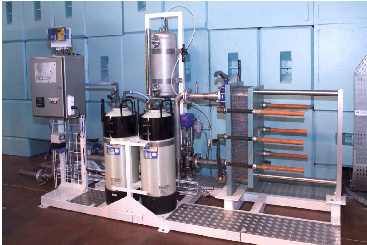
Beam stopper cooling system
