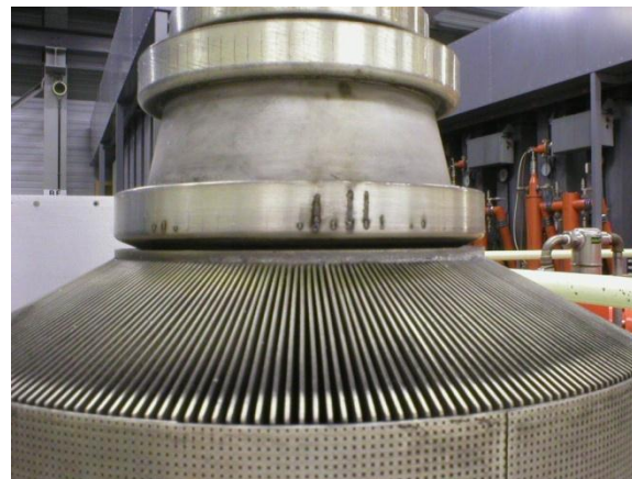
Philips burnt tube because of lack of air cooling
