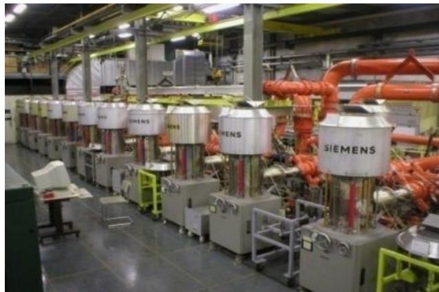
20 x 135 kW RS2004 'Siemens' plant (1976 to 1979)
