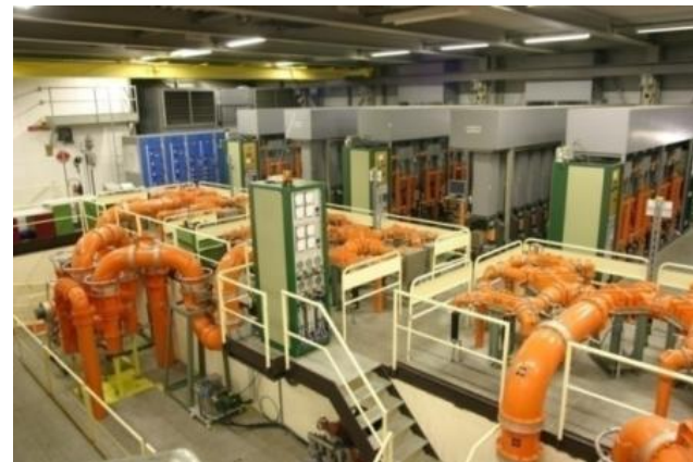
68 x 35 kW YL1530 'Philips' plant (1980)
