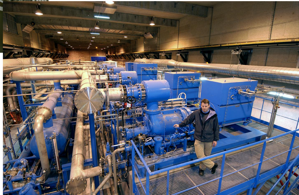
Oil-injected screw compressors at LEP2 (1996)
