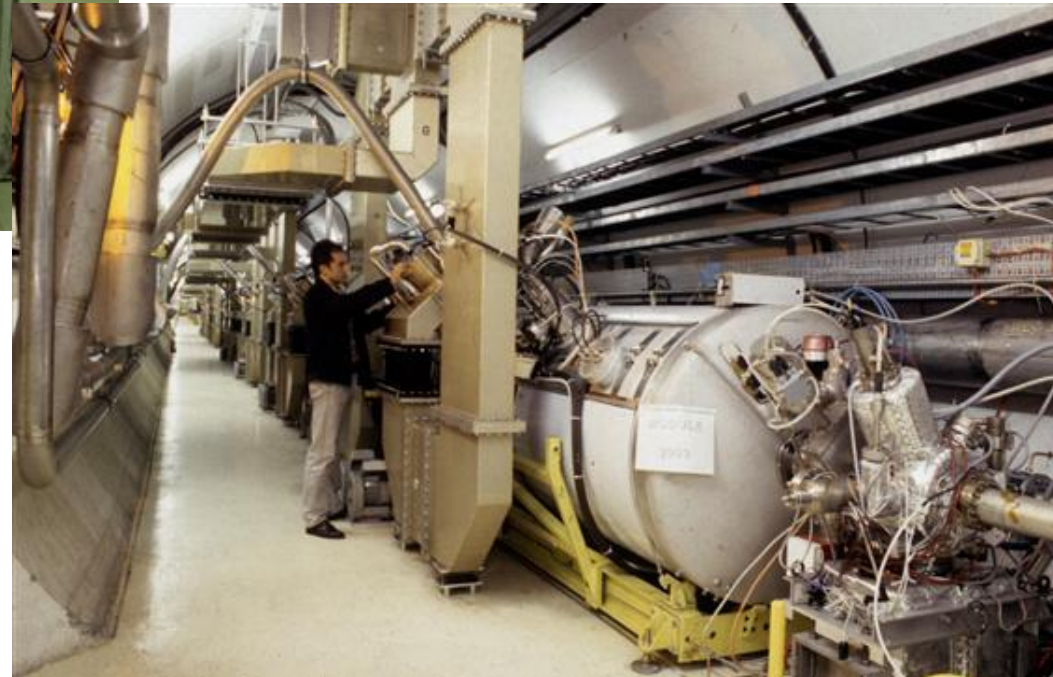
Cryomodule in LEP tunnel
