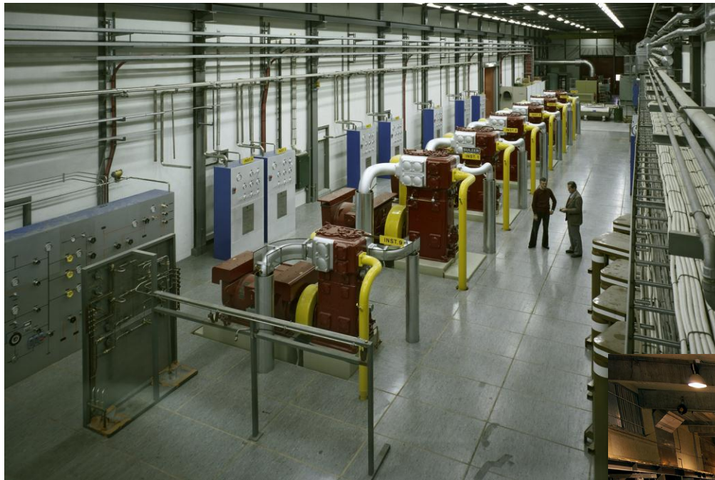
Sulzer piston compressors in North Area (1977)
