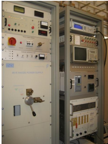
20 kV PSU & Aux. rack – front view
