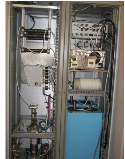
38 kV PSU – rear view
