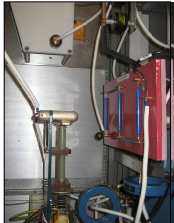
38 kV PSU Dump Relay & Voltage divider
