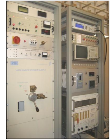
20 kV PSU and Aux. Rack
