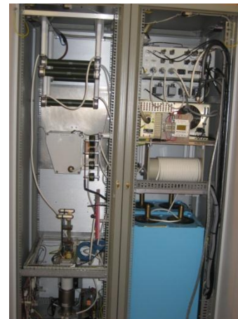
38 kV PSU - rear view
