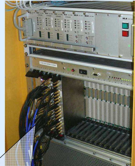
E-XFEL cavity BPM electronics for 2 BPMs (works in MBU and standard VME crates)
