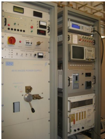
20 kV PSU & Aux. rack - front view
