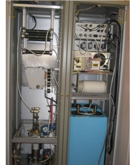
38 kV PSU – rear view
