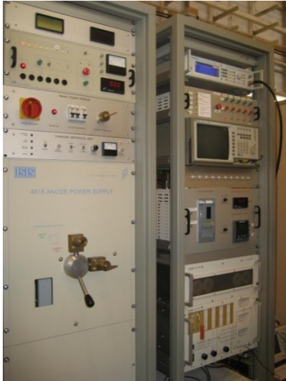
20 kV PSU & Aux. rack – front view
