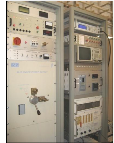
20 kV PSU and Aux. Rack
