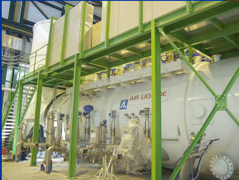
Air Liquide cold box
