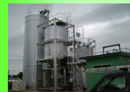
Water treatment system
