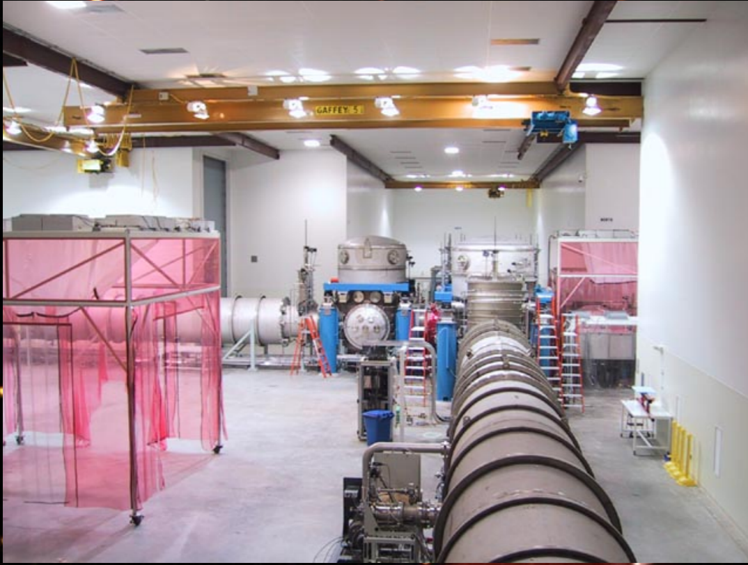
Vacuum system inside the corner station at Livingston
