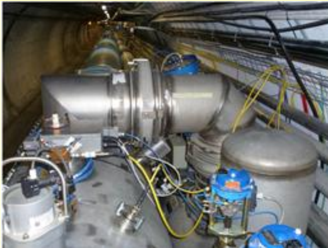
A19R3 Jumper. Leak on the weld 4.10^{-4} mbar.l/s Temporarily fixed with mastic until LS1
