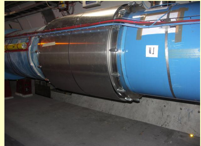
A15L4.M Leak on seal 3.3.10^{-4} mbar.l/s (risk to repair leak : No action until LS1)
