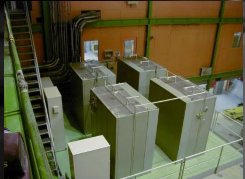
Four HVPS for SPS 352 MHz tetrode amplifiers
