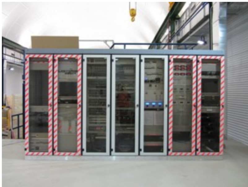
PLC Slow Control System
