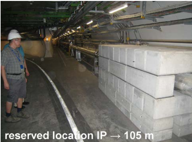
Figure 48: Concrete shielding block installed in the LHC tunnel close to the reserved wire-compensator location [photo R. Steinhagen].
