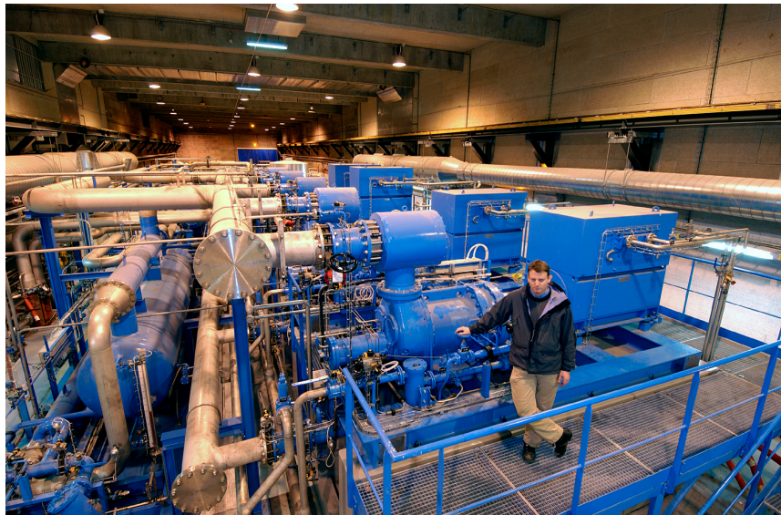
LHC 1.9 K cryo plant
