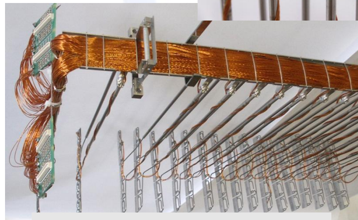
Cable channel with sensor cables
